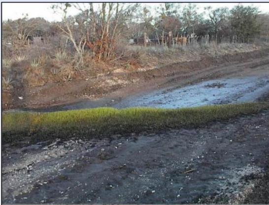
Compost filter berm, US HWY 281 (Texas) on 1/30/2001
