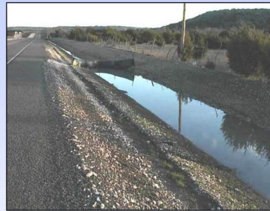
Silt fence, US HWY 281 (Texas) on 1/30/2001
